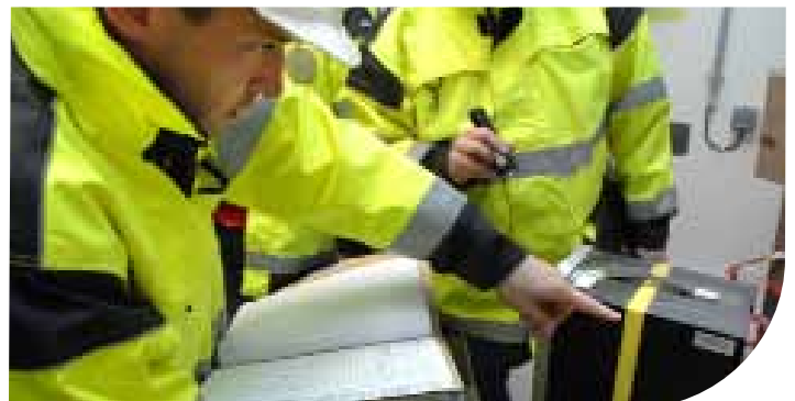
Fire Water System: First Pressure Test
